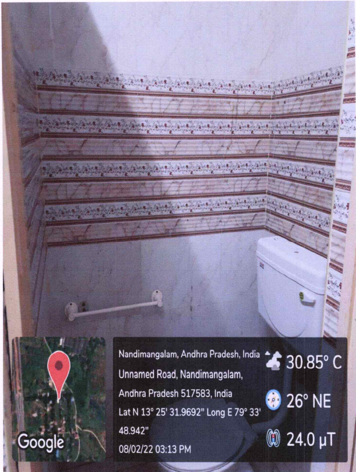
Fig: Provision for Washrooms for differently abled people in the college campus
